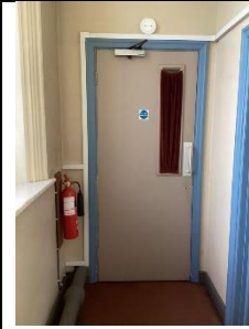
Figure 33 Typical fire door which could be upgraded to a modern standard
