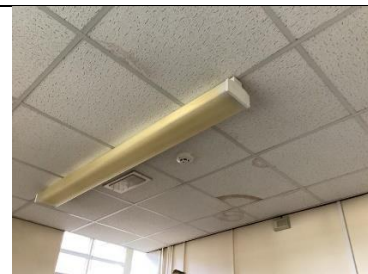
Figure 39 Example of fluorescent lighting
