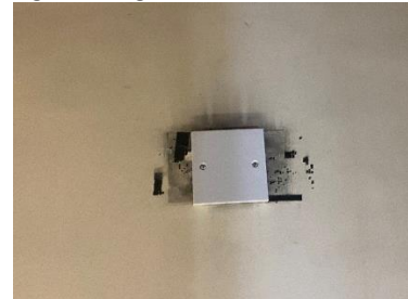
Figure 38 Failed socket outlet
