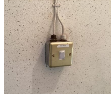
Figure 37 Light switch with MICC feed
