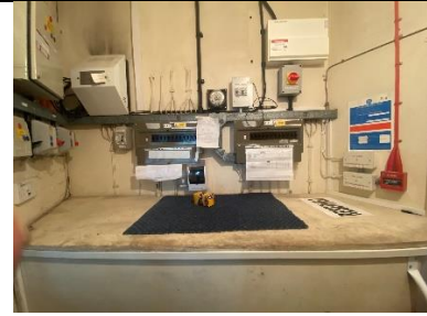
Figure 36 Example of switchgear
